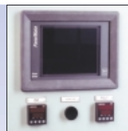
Programmable Logic Control System (PLC)
