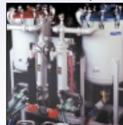
Raw material day tanks
