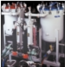
Raw Material Tanks
